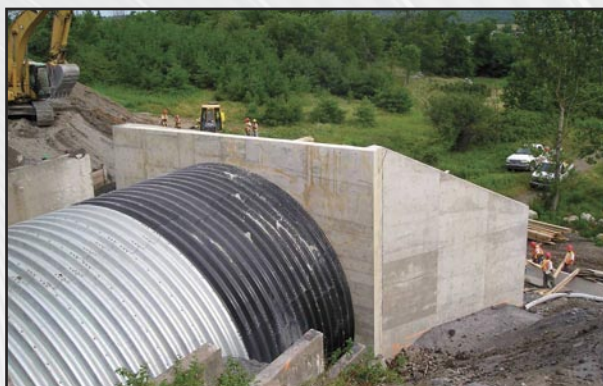
Vehicular Underpass with Top Plates Polymer Coated for Deicing Salt Runoff from Major Highway
