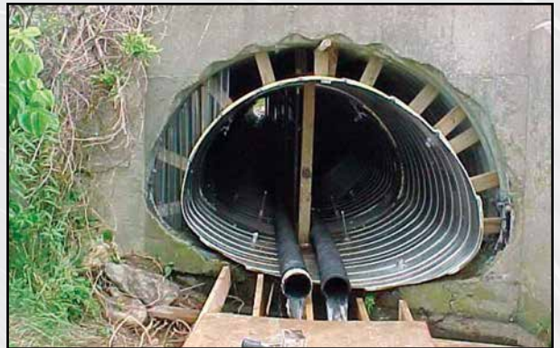
BYPASS PIPING AND END BRACING
