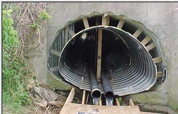
BYPASS PIPING AND END BRACING
