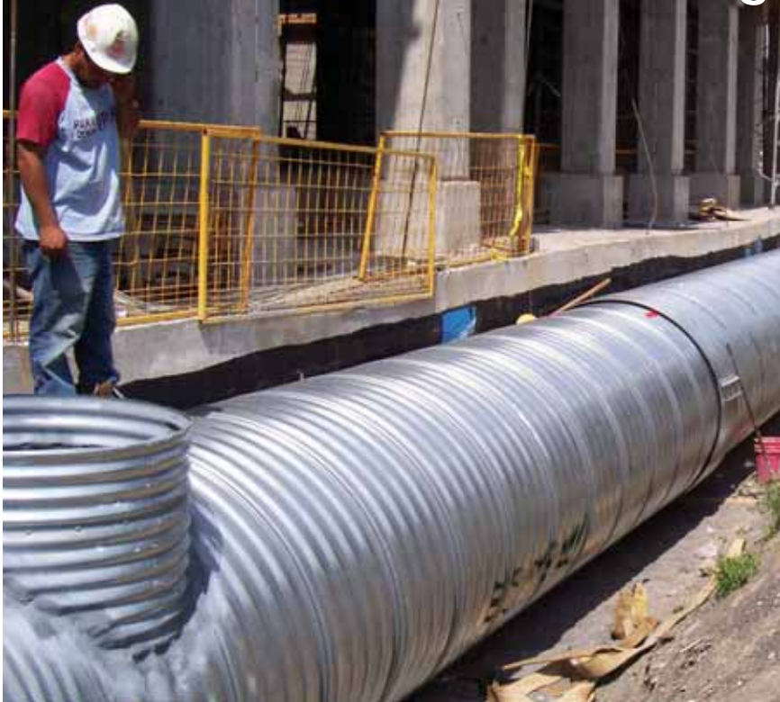
1700 mm diameter CSP stormwater detention tank below One Park Tower.
